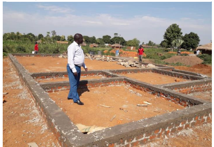
DAO supervising construction works at BInagoro women's group, Midigo Sub county, Yumbe district
