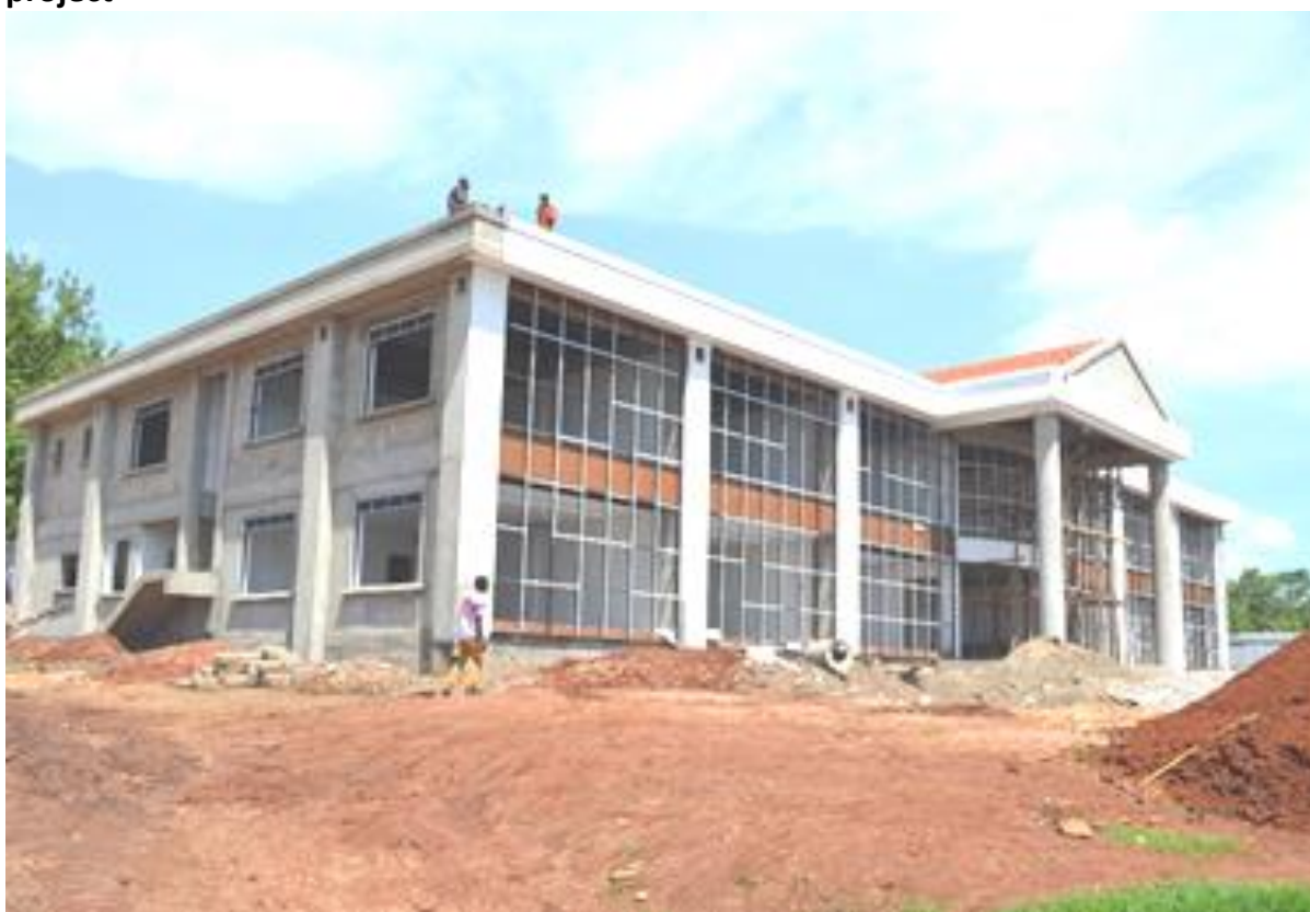
Figure 23: The Cassava Regional Centre of Excellence under construction by the EAAPP project
